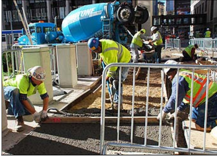
Workers for YAW Construction pour sidewalk in front of the federal courthouse at Fourth and Robert streets as part of the utility relocation work in downtown St. Paul.
